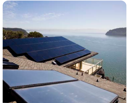
Rooftop solar PV and solar water.
